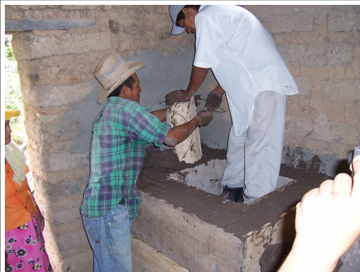
Placing chimney tiles on top of metal can and wrapping barb wire around tiles to hold in place
